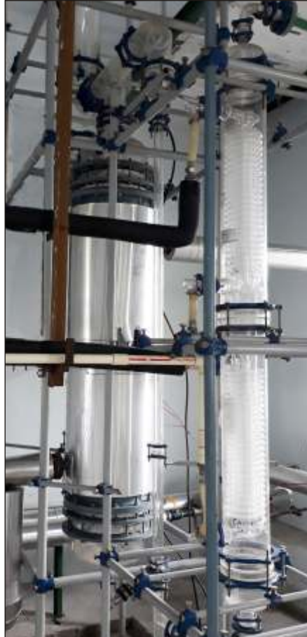
HCL GAS GENERATOR
